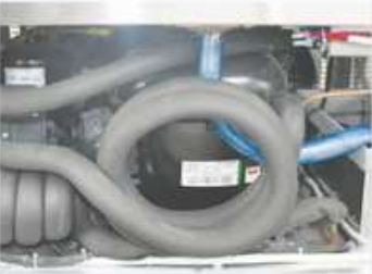
Cooling System High power Cooling System
